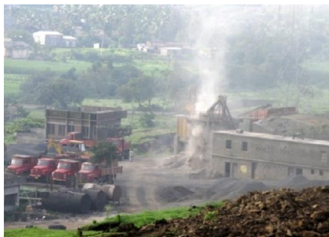
Fig. 4 Crusher emitting dust near village Top
