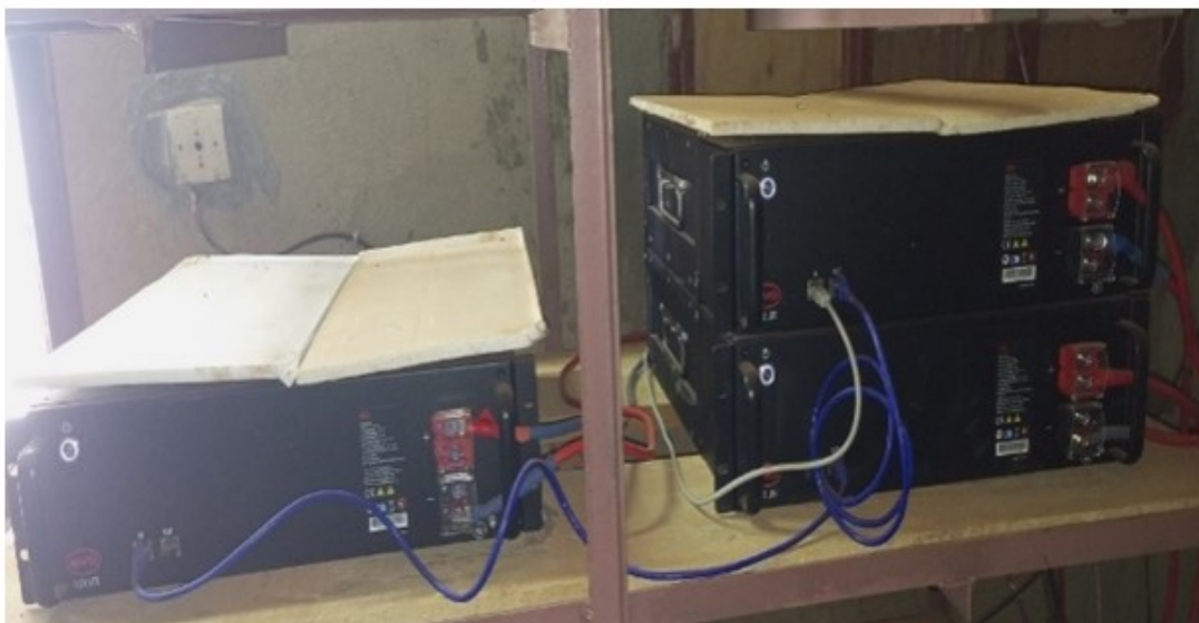
Figure 8. Lithium battery park of site
