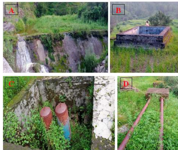
Plate 3. Typical example of hydram infrastructure of Chan Hydram in the Upper Kosi watershed: A- Check Dam, B- Water Storage Tank, C- Hydram Pump and D- Pipeline
