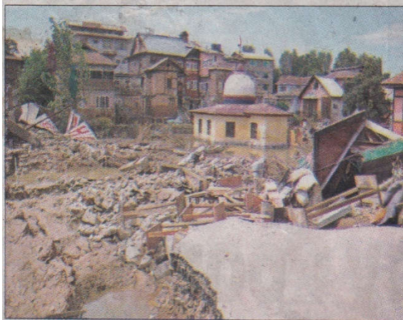
Abiguzar bund stands cracked.
