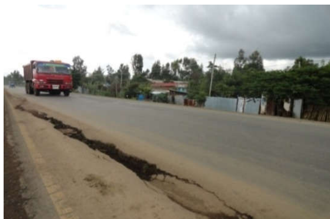
Fig. 2. Cracks on Ambo–Addis Ababa road
