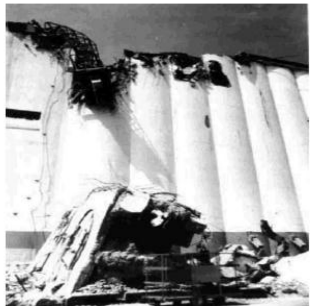
Fig. 1. Partial collapse of grain silo during 1974 Lima, Peru earthquake
